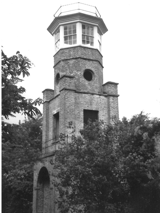
Fig.1. Thomas Oldham's prospect tower during restoration, after the lantern top was fitted, but prior to windows being installed.
