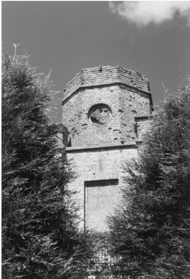
Fig. 5. The prospect tower, south elevation prior to restoration (1999). Remains of the painted glazing bars can be seen in the blank window.
