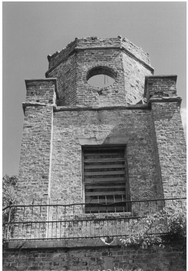
Fig. 6. The prospect tower, west elevation prior to restoration (1999). Yorkstone strings and window lintel; railings with acorn finials. The square pillars were originally topped with Yorkstone urns. All these features are shown in Thomas Espin's 1815 Louth Town Hall design.
